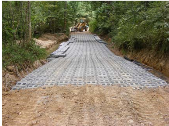
The hardened stream crossing helps reduce erosion and provides a sustainable surface.
