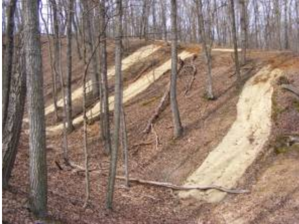
Part of the area repaired with money received from grants and a lot of help from volunteers.
